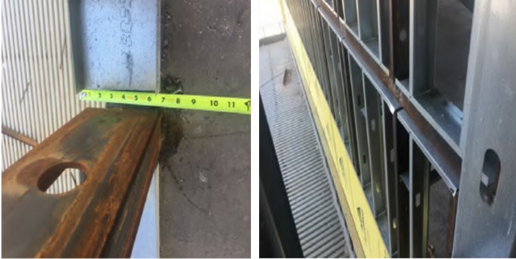
Figure 5. Photographs of the stud track (left) and stud wall (right) overhanging the edge-of-slab.
