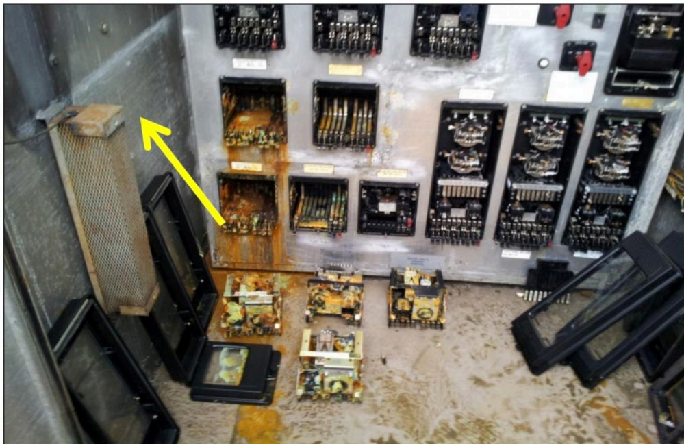
Figure 11. Photo published by Con Edison of protective relay equipment damaged by flooding during Sandy at Con Edison facilities. Yellow arrow indicates horizontal water mark suggesting maximum flood water level at this location.
