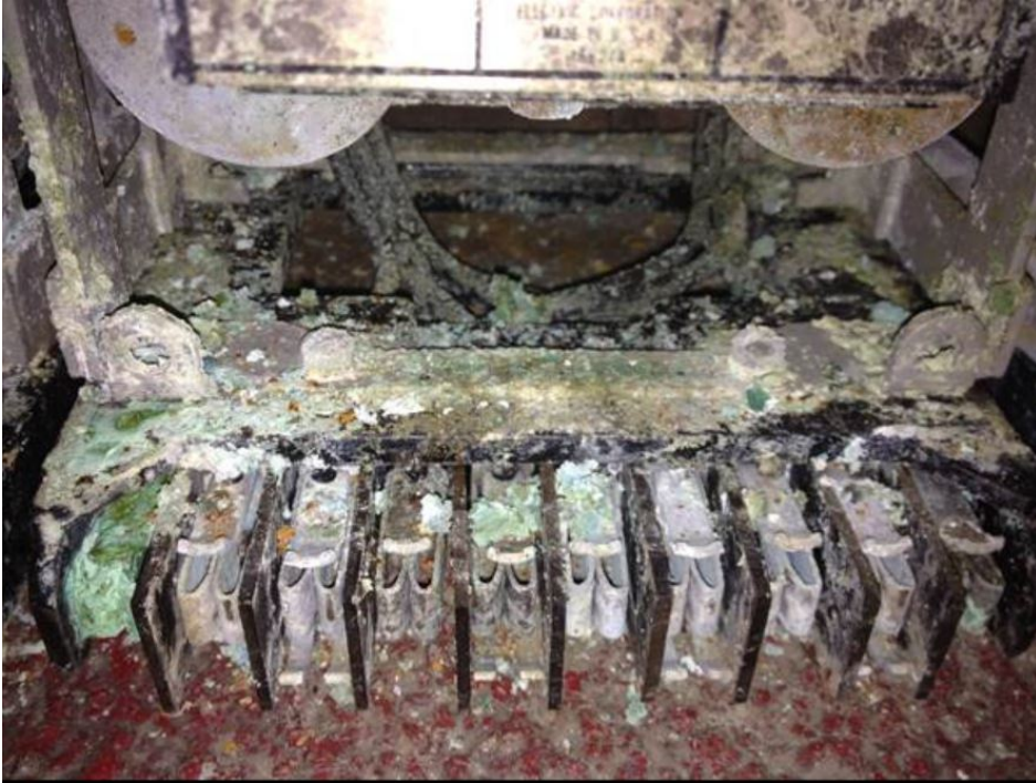
Figure 10. Photo published by Con Edison of protective relay equipment damaged during flooding at East River Complex during Sandy.
